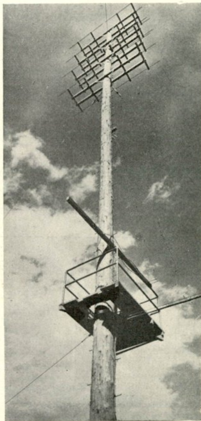
Elaborate High-Frequency Antenna System used by Bell Telephone Engineers.
