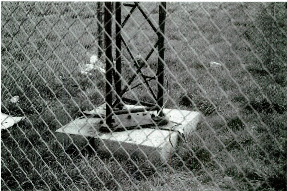
photo 4.5 – This slant wire fed AM tower is grounded through the copper straps across the base pad. The wire leading from the right leg of the tower supplies AC power to the obstruction lights.
