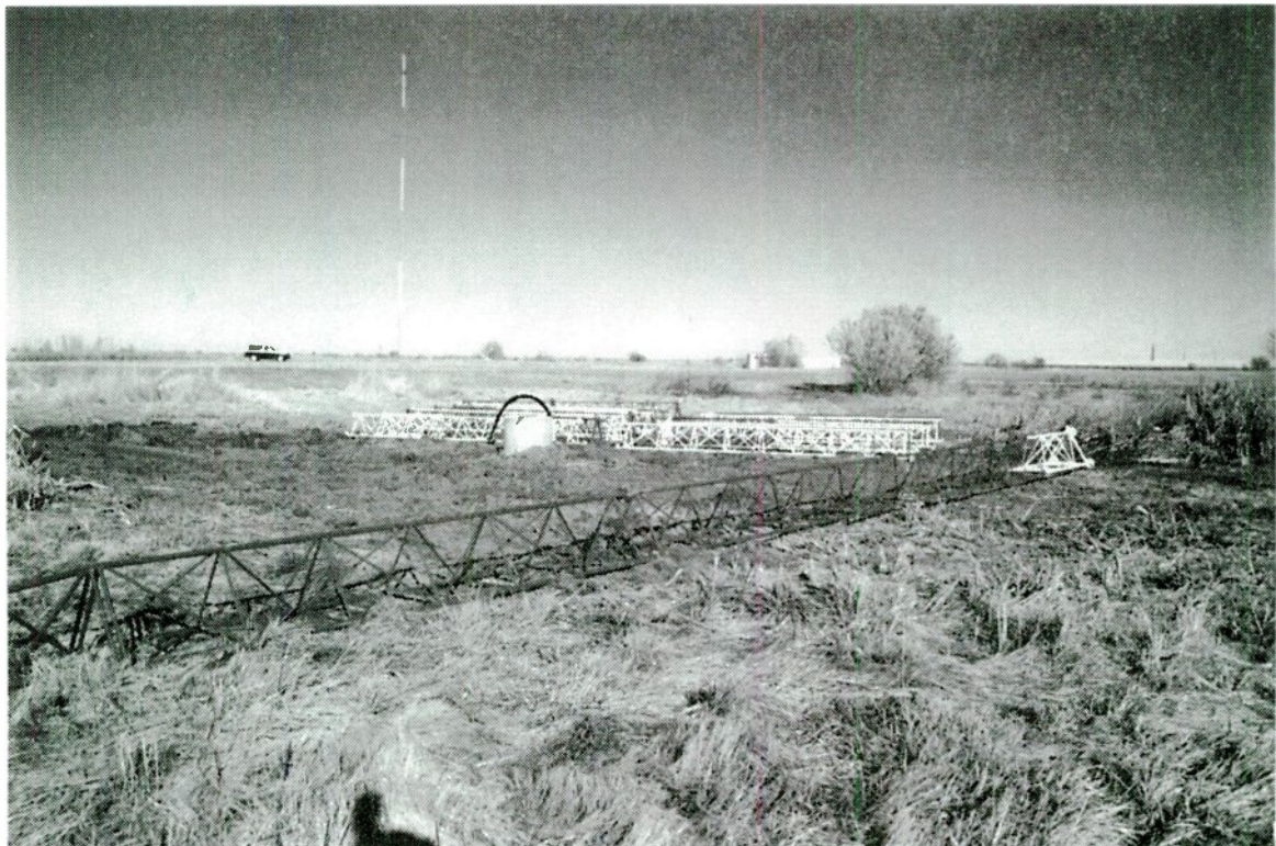
photo 6.12 – Sections of a new tower await installation as another tower in the background nears completion.
