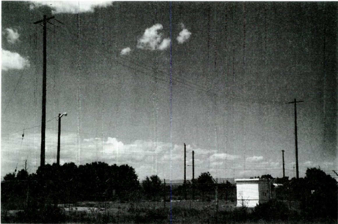
photo 4.1 – This classic ‘flat top’ style antenna is a ‘T’ configuration. It is currently in use as an aircraft navigation beacon operating near 400 kHz.
