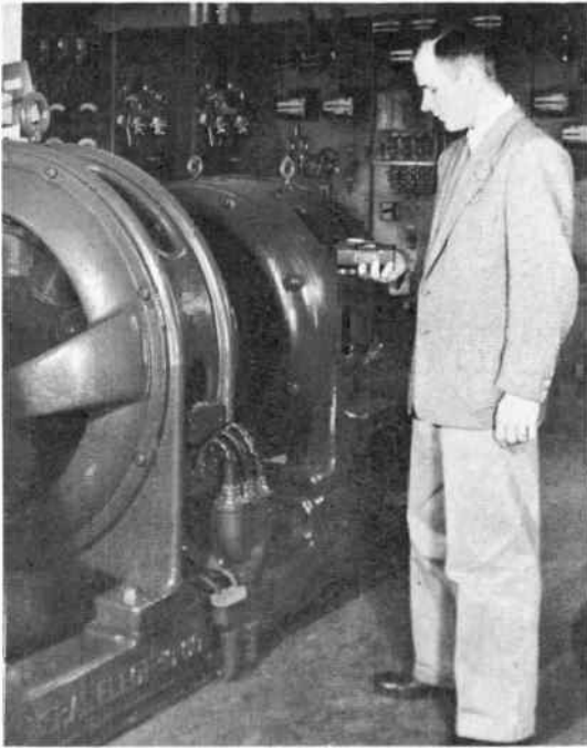
Figure 5-2. The Sound-Survey Meter being used to measure noise from rotating electrical machinery.
