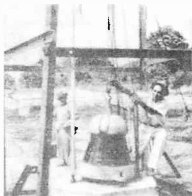
FIG. 2.62. The first step in the construction of a guyed vertical radiator for broadcasting—setting the base insulator. This photograph was taken in Peru. (Photograph courtesy of R. E. Lee.)
