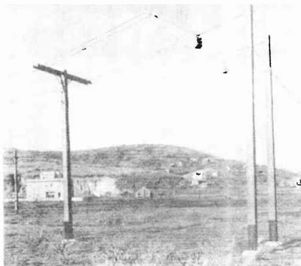
FIG. 4.86. Details showing a terminal pole for two balanced two-wire feeders and the manner of maintaining constant tension on the vertical feeders for a beam antenna. These methods were used for transmitting 50 kilowatts for high-frequency broadcast service. The station building can be seen in left background. (Photograph courtesy of Radio Nacional, Rio de Janeiro and RCA International Division.)
