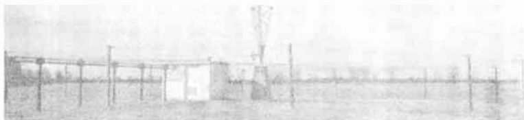
FIG. 1.16. Ground screen for a vertical radiator. (Photograph from Radio Station KTBS, courtesy of W. M. Willy.)
