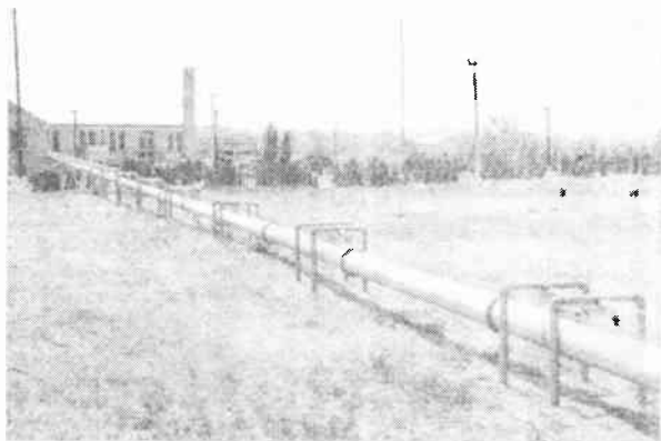
FIG. 4.75. View of a 10-inch coaxial feeder built for Station WJZ in 1937 and designed for 2,000-kilowatt peak power transmission. The feeder is straight and is free to expand and contract with temperature changes. The flanges on the feeder mark the length of each section and the location of the insulator supports for the inner conductor. (Photograph courtesy of National Broadcasting Company.)
