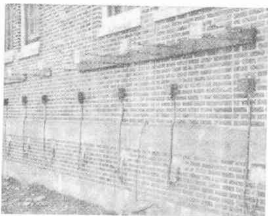
FIG. 4.106. Detail showing the feeders for a receiving installation using four-wire cross-connected open-wire feeders terminating at a building and entering through coaxial feeders. The wide-band high-frequency balance to unbalance transformers are in the weatherproof black boxes on the building. (Photograph courtesy of Royal Canadian Navy.)
