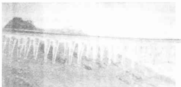
FIG. 1.42. Example of heavy icing on an antenna wire. (Photograph courtesy of J. S. Hall and C. I. Soucy.)
