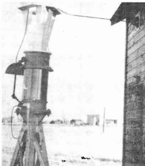
FIG. 2.64. Base insulator of the Austin oil-filled safety-core type with the tower-lighting transformer located inside the base insulator, at Station CKLW. (Photograph courtesy of RCA Victor Company, Ltd., Montreal.)
