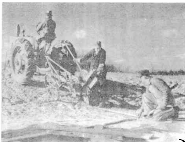
FIG. 267. A tractor-drawn wire plow for burying ground wires. The plow blade is sheet steel that cuts a thin furrow. The wire is fed into the furrow as the plow advances. Horse-drawn hand plows of similar principle are often used.
