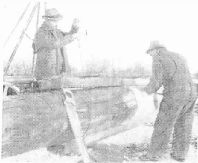
FIG. 3.112. The beginning of a pole-splining operation and the construction of a butt-spliced pole. (Photograph courtesy of National Broadcasting Company.)
