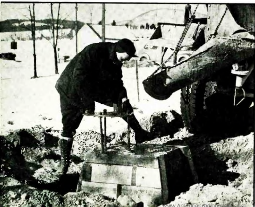
Fig. 8. The assembled base plate and anchor bolts, ready to put in place
