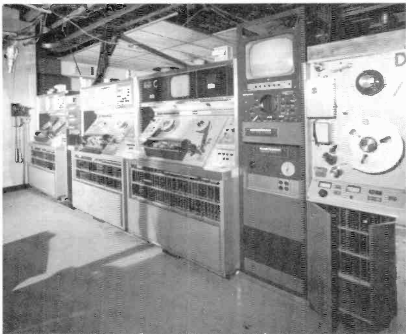
Fig. 8-21. VTR room at WTAE-TV.
