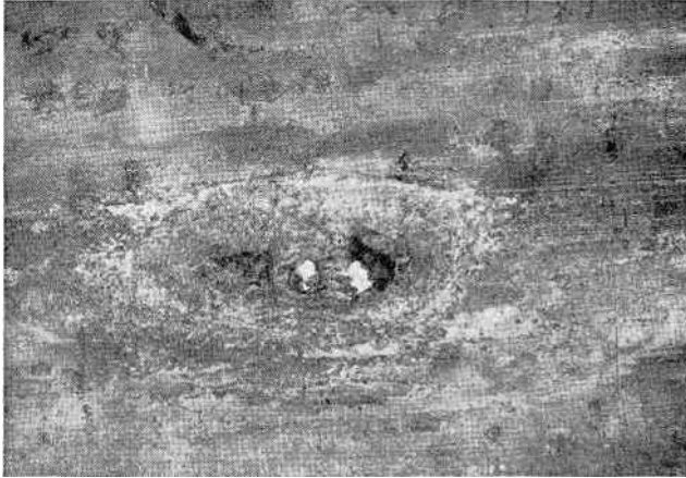
FIG. 57.—Damage done by electrolysis to a lead cable sheath. ( Courtesy of Bell Telephone Laboratories. )
