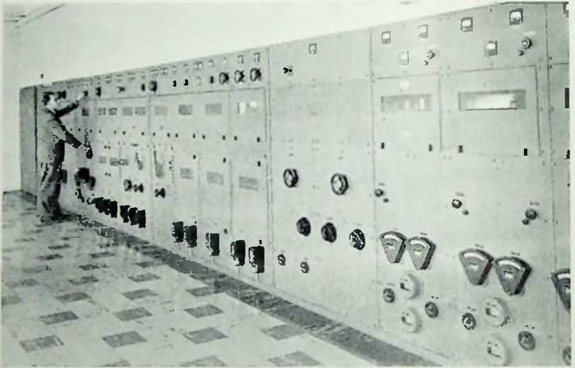
FIG. 1.10c. MAIN TRANSMITTER FOR G-E TELEVISION BROADCASTING STATION WRGB, LOCATED IN THE HELDERBERG MOUNTAINS, NEAR SCHENECTADY, N.Y.
