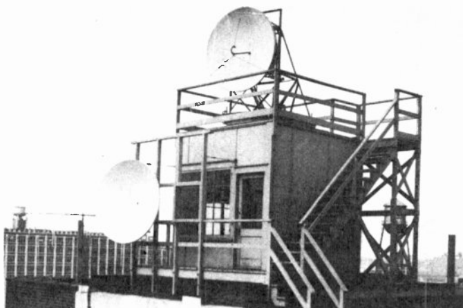
Figure 104. Permanent installation of microwave relay antenna.
