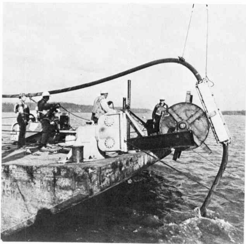
Figure 2-13 Installation of a coaxial cable in the Mississippi River. Bell Labs Photo.
