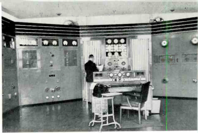
Control room at WNBC's transmitter, Port Washington, Long Island
