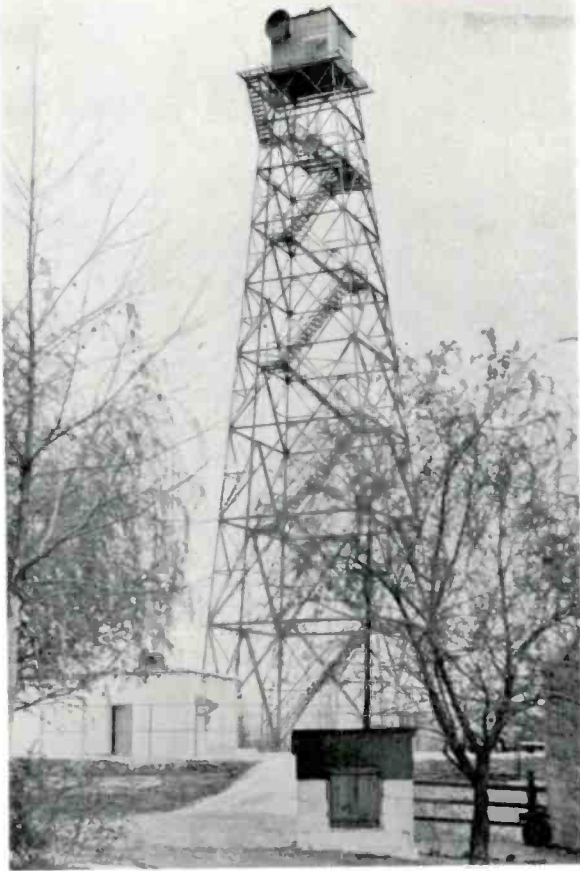
Automatic radio relay tower used to transmit television signals from point-to-point.
