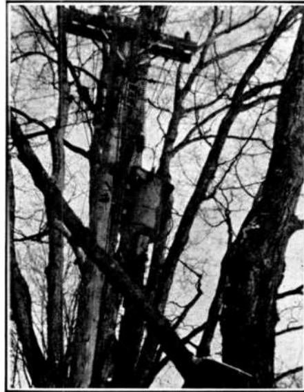
FIG. 87. Careful trimming of trees is required to avoid tree grounds and consequent interference.
