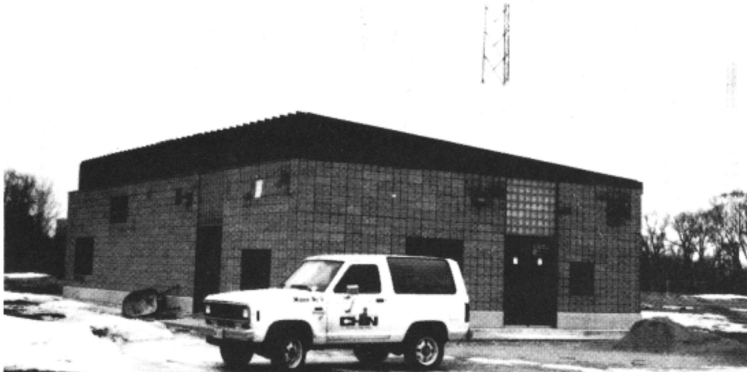
Photo 4: Transmitter building, of block construction, has 70-year-old concrete bins as primary foundation.
