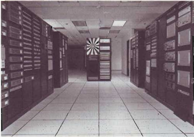
TQS Central Equipment area.
