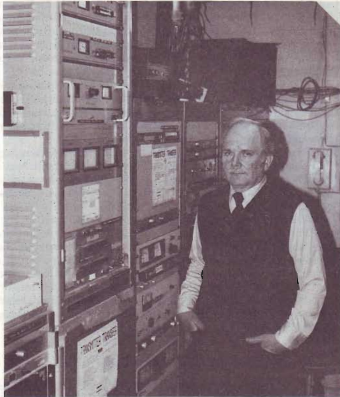
Fred Cole at CKDA's transmitter building during normal operations.
