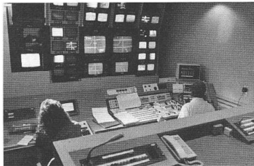
The new CFRN-TV control room
