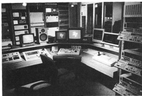
CISA-TV's ACE edit suite has all the bells and whistles needed for the station's heavy local news, sports entertainment and community programming.
