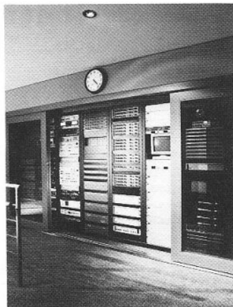
Rack wall outside engineering.
