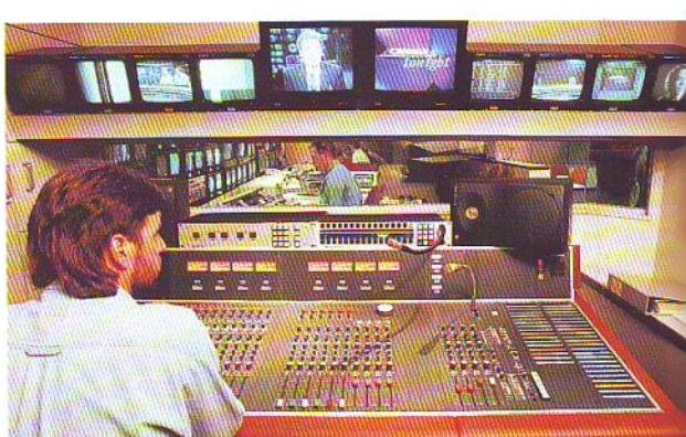
New CHCH-TV News audio control centre. In background are primary technical/production work stations.
