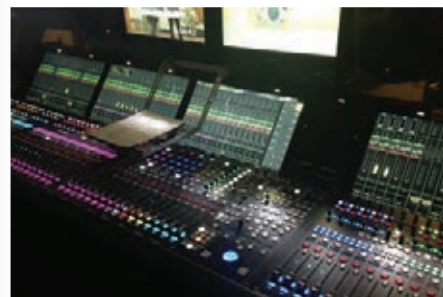
Shopping channel QVC has had new audio consoles and central routers installed in its broadcast facilities, in a major project handled by Lawo out of Toronto.
