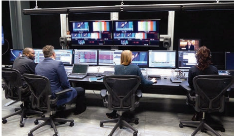
Inside the new playout facility provided by ATG Danmon for Trinity Broadcasting Network UK and Europe.
