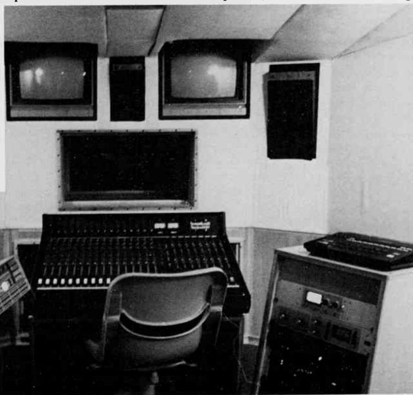
A view of the studio control room, showing the electronic keyboards, console and audio/video monitors. (Inset) The reflection-free zone created by the special panel, which was designed and patented by Dr Peter D'Antonio.
