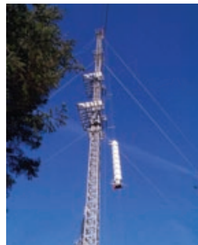
DCENR has continued its Digital Terrestrial Television (DTT) trial service from the RTÉNL transmission sites at Three Rock and Clermont Carn.
