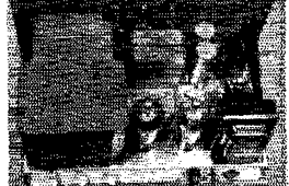
Dual Power Supply Section
