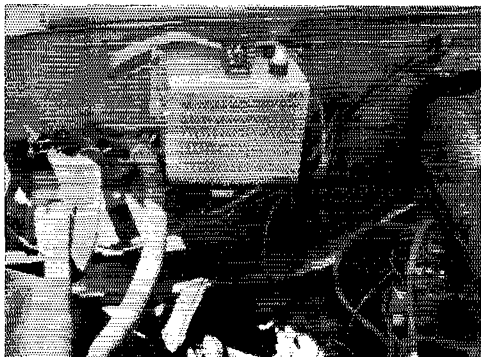
The a.c. inverter installed on the fire wall of the author's car.
