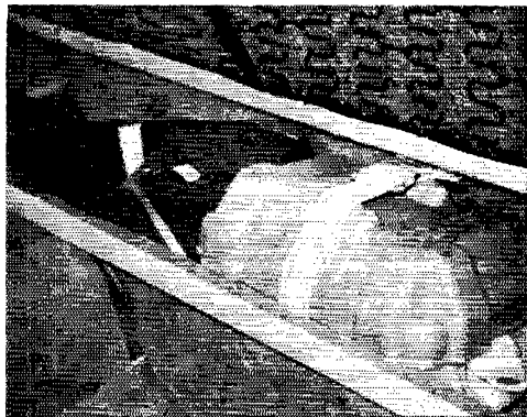
Fig. 2—The auxiliary 12-volt battery is mounted under the left rear seat in a plastic battery box.
