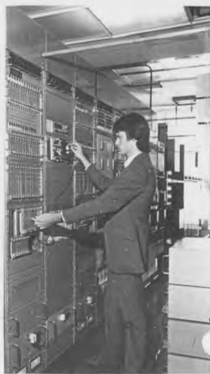
PCM coder in London Control Room
