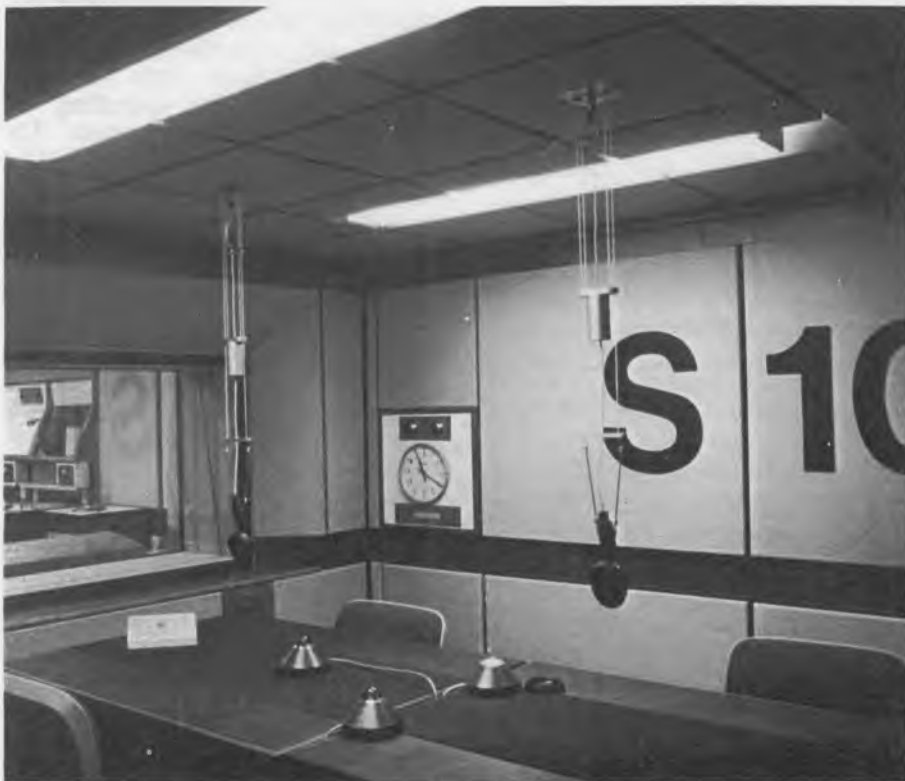
A typical Bush House Talks Studio, S10. Note the counterbalanced microphones (designed specially for External Services) and the differing finishes of the table top, leather for writing and baize for absorbing the sound
