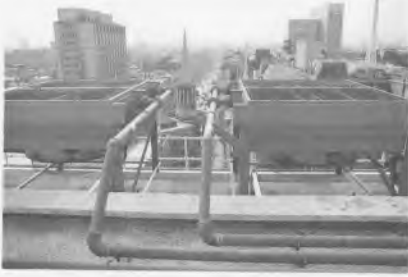
Engine Radiators on roof of Broadcasting House Extension 13 floors above the generators.
