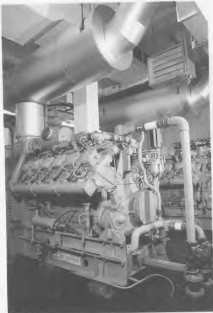
474kW turbocharged V12 generating sets in BH sub-basement engine room
