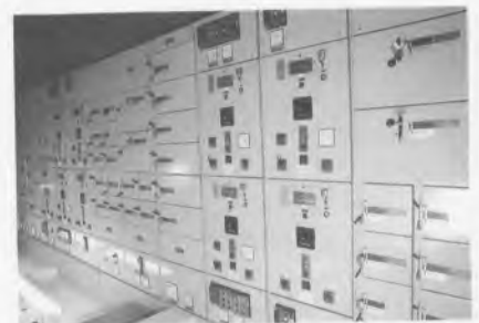
New Maintained supplies switchboard
