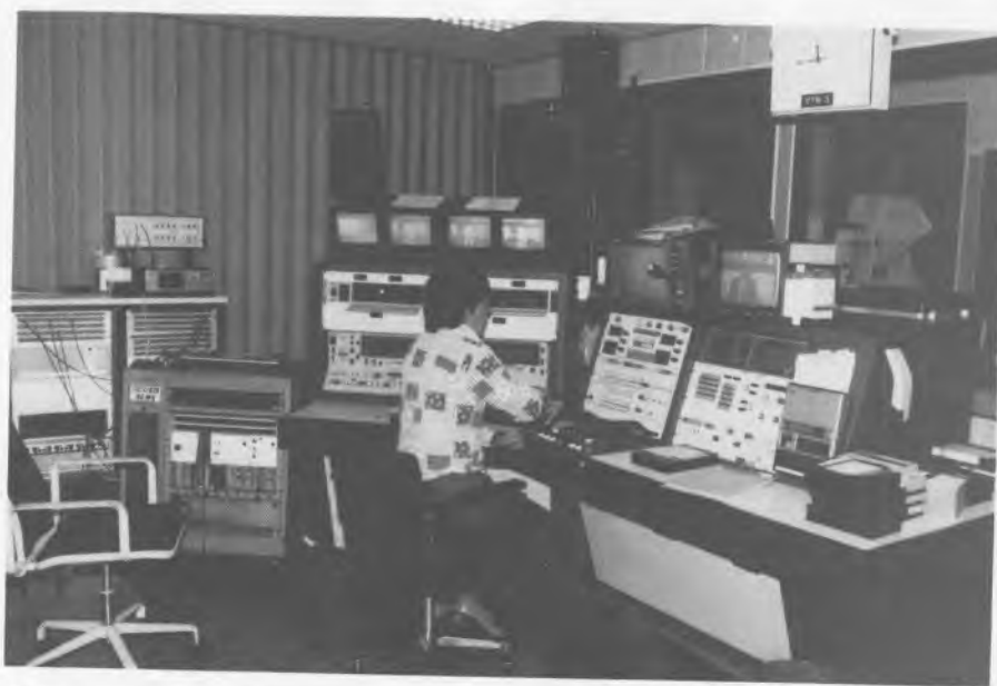
VTN 1 - one of two identical C-format transmission cubicles with Roy Osborne at the control desk
