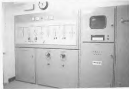
System control panel containing GEM-80 and showing the operational mimic diagram, VDU and printer.
