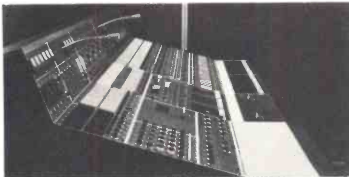
Neve 24-channel console installed at Nova Sound Studios
