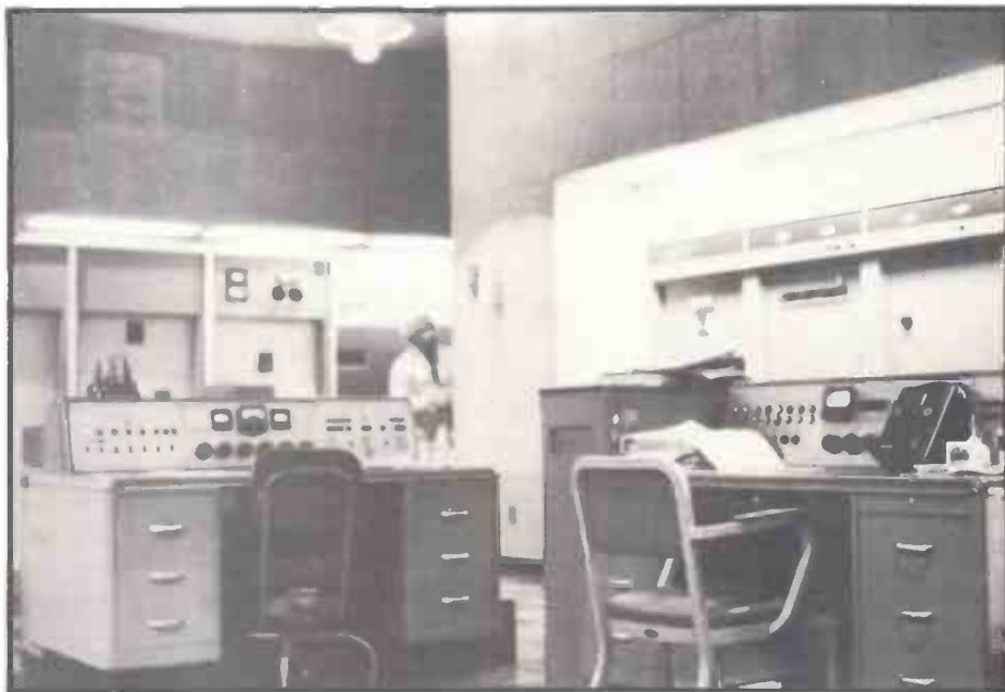
Transmitter room with Gates MW-50 (right) and RCA transmitter (left)
