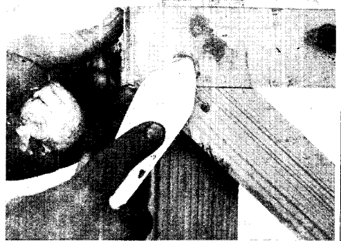
Fig. 3. Large holes such as those made by nails should be filled in with hard stopping or putty
