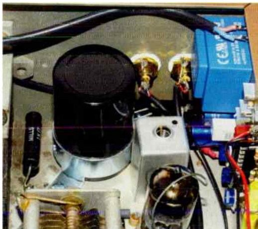
Soldered joints should be sleeved and the cable secured, for safety.
