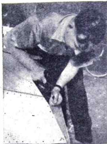
Shaping off the bows of a ply-skinned boat. Edges of the ply are trimmed off flush and the pointed bow proper is shaped from a block of wood which is then glued and screwed in place
