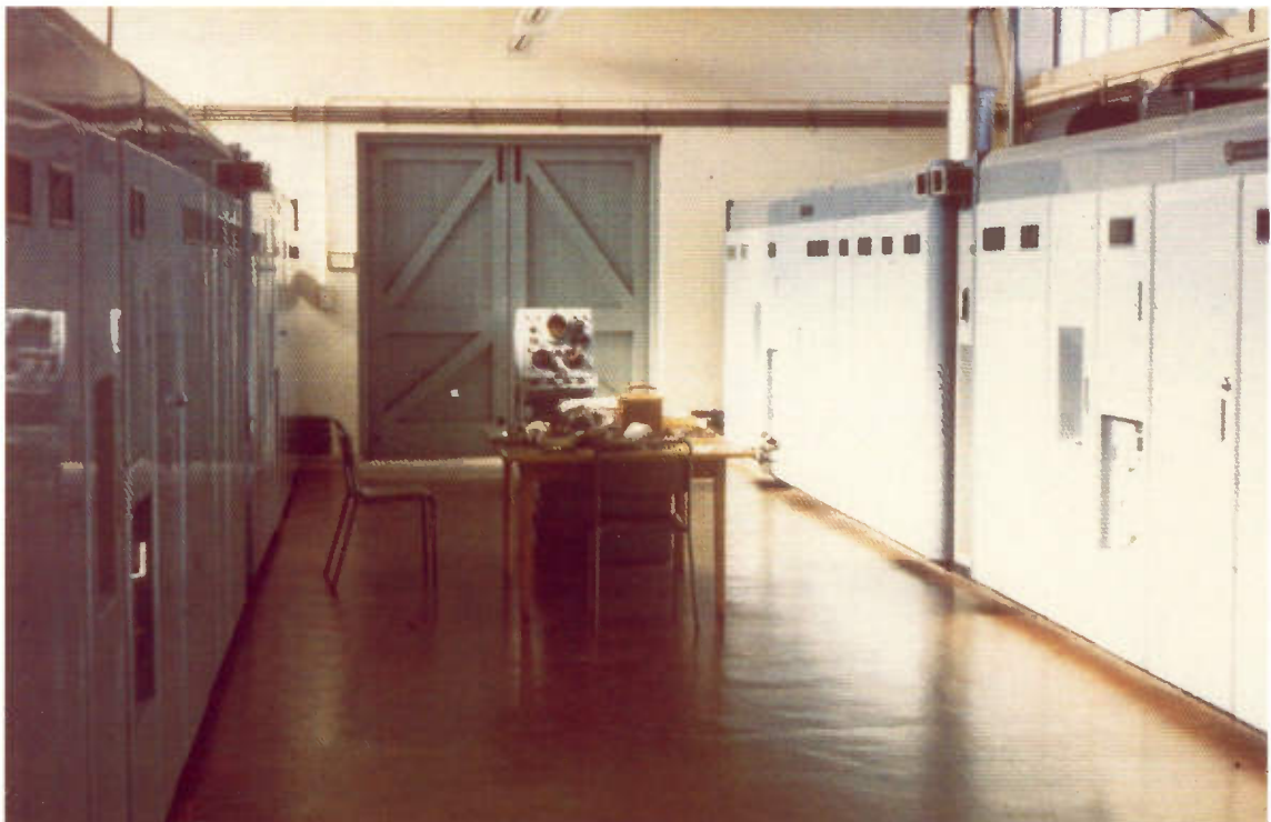
S.T.C. 30kW Transmitters in 'B' Station
