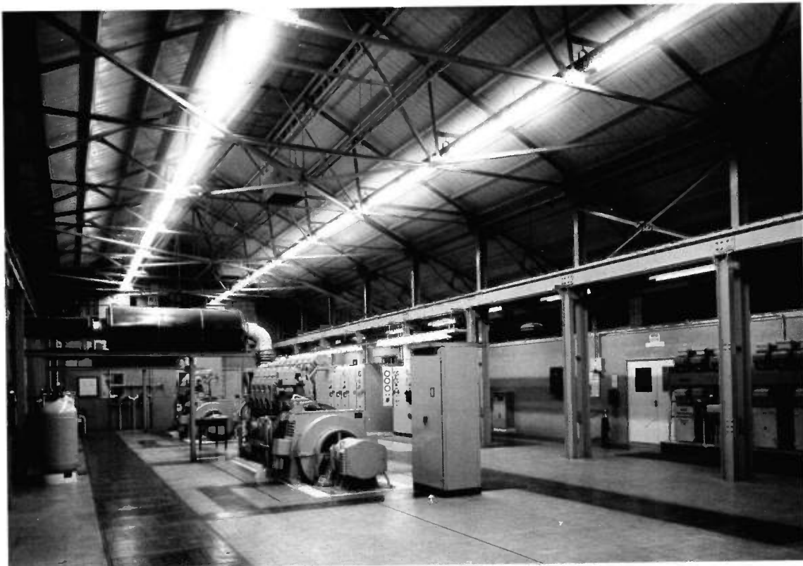
The Power House with the New English Electric Generators
