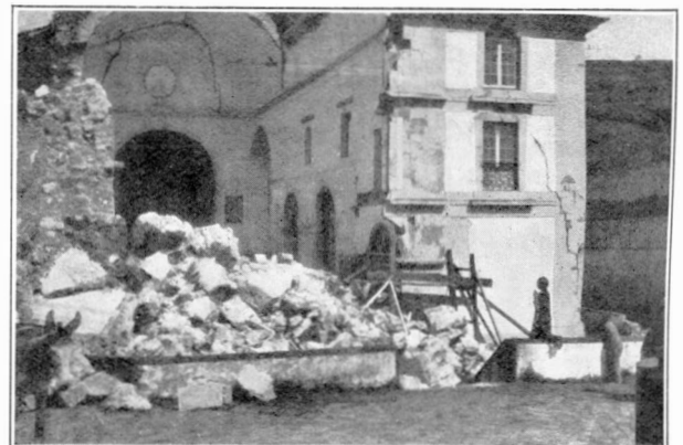
FIG. 9.—DAMAGE DONE TO CHURCH BY EARTHQUAKE.
