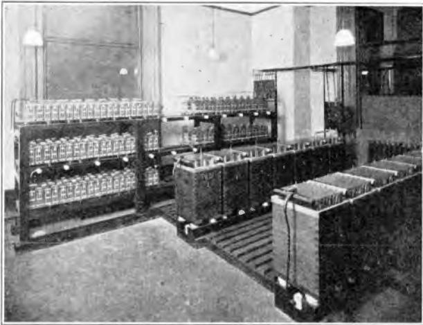
FIG. 2.—FILAMENT AND ANODE BATTERIES.
