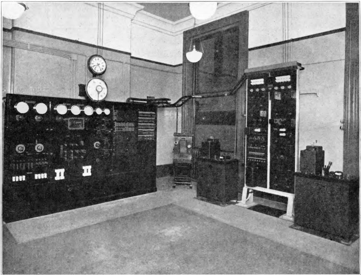
FIG. 1.—POWER SWITCHBOARD, SENDING MACHINE, CONTROL RACK, RECEIVING MACHINE.
