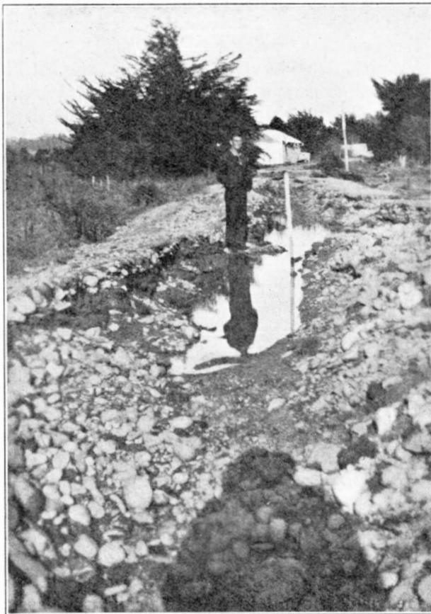
FIG. 11.—KARAMEA. RUINED ROAD WITH FISSURE FILLED WITH WATER.
