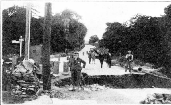
FIG. 2.—SUBSIDENCE NO. 2. VIEW FROM SOUTH EAST.
