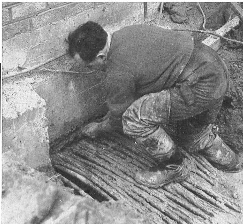
24 1/2" diameter cables passing through duct measuring 36" x 18" x 9" which is completely filled with DENSO MASTIC.
