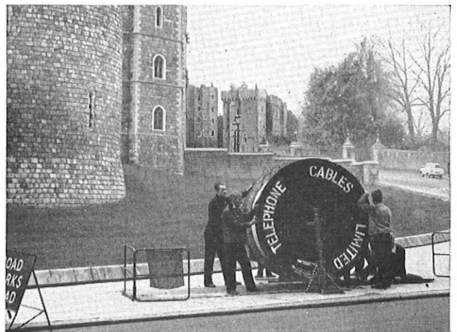
T.C.L. moisture barrier cable at Windsor Castle.
