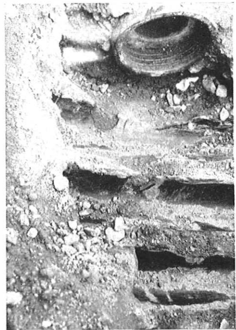
DAMAGE TO DUCT ROUTE CONTAINING HIGH WYCOMBE-LONDON No. 2 CABLE
