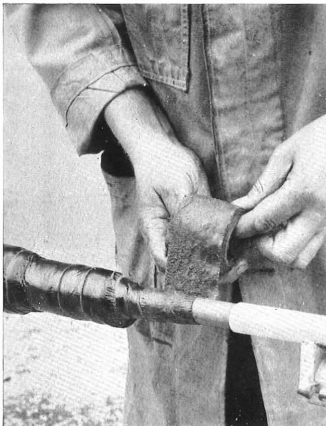
Tape Sealing No. 3 (DENSOPOL ZN) being used to protect a joint in thin lead sheathed, polythene oversheathed cables by the G.P.O. Experimental Jointing Division. Winn & Coales Ltd. have been suppliers to the Post Office of waterproofing and anti-corrosion tapes for over 25 years.
