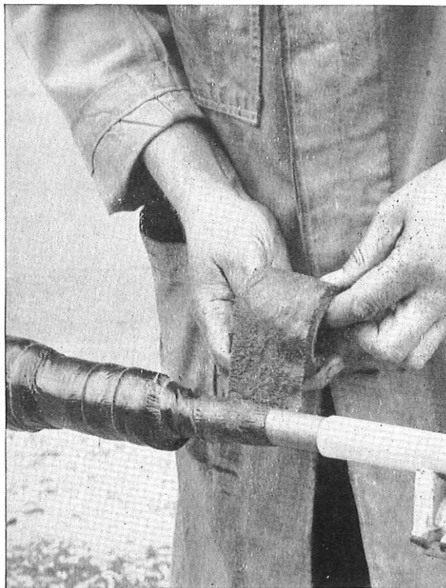
Tape Sealing No. 3 (DENSOPOL ZN) being used to protect a joint in thin lead sheathed, polythene oversheathed cables by the G.P.O. Experimental Jointing Division. Winn & Coales Ltd. have been suppliers to the Post Office of waterproofing and anti-corrosion tapes for over 25 years.
