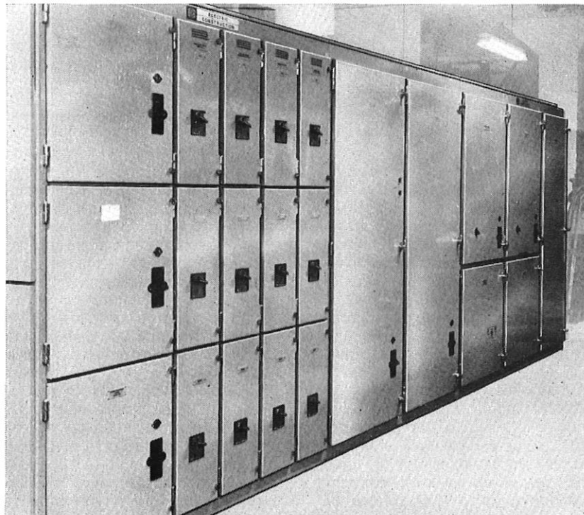
FIG. 4--PLANT NO. 1 AUTOMATIC CONTROL AND DISTRIBUTION CUBICLE
