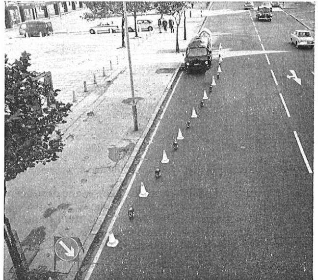
FIG. 4—Layout of guarding equipment: plant in the carriageway; day and night working
