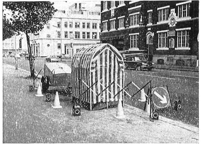
FIG. 3—Layout of guarding equipment: plant in the footway; day and night working
