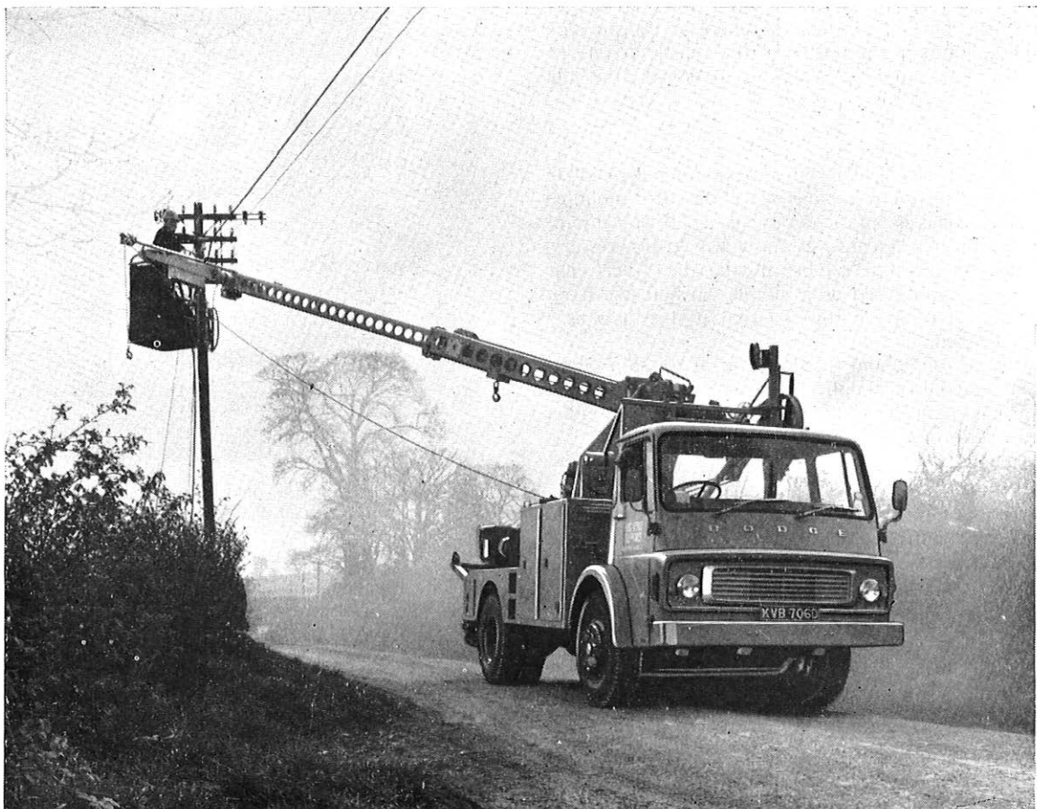
FIG. 5—Aerial-cabling unit erecting replacement cable for an open-wire route using the “drawing-in” method
