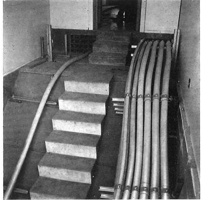
FIG. 4—M-type cable pit showing cable slope and access under the raised floor in the m.d.f. room
