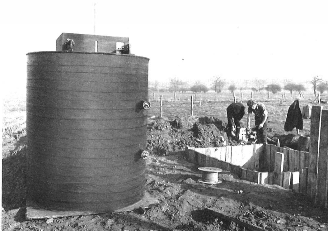
FIG. 4—The silo buried repeater station
