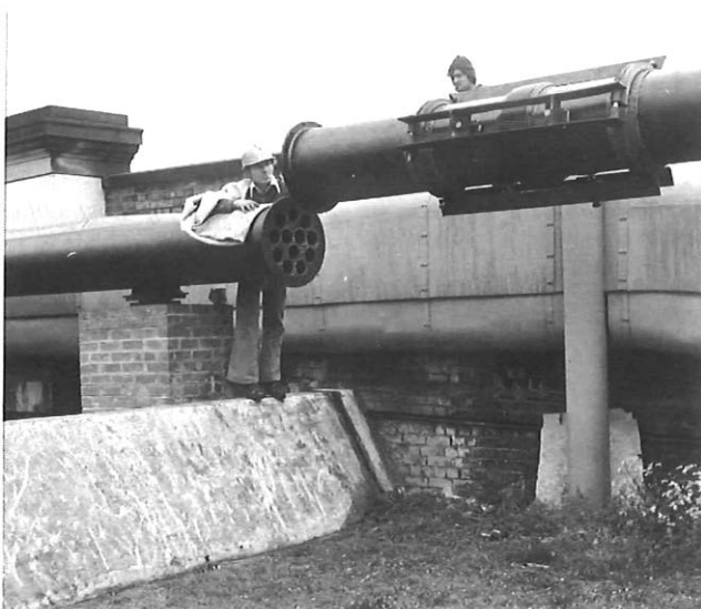
FIG. 2—Pipe-work at the eastern end of the bridge, showing the bellows section
