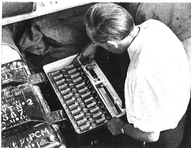
FIG. 4—Installation of a 24-channel PCM system
