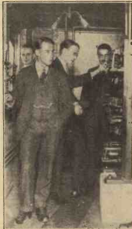
Mr. Rogers (left) and Mr. Dowding (at switchboard) in a corner of the "P.W." workshop.
