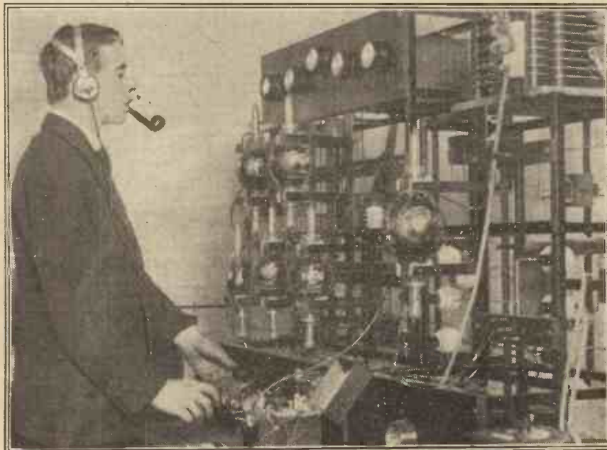
Mr. H. P. Cook, assistant engineer of the Hull Relay Station, tuning the transmitter.
