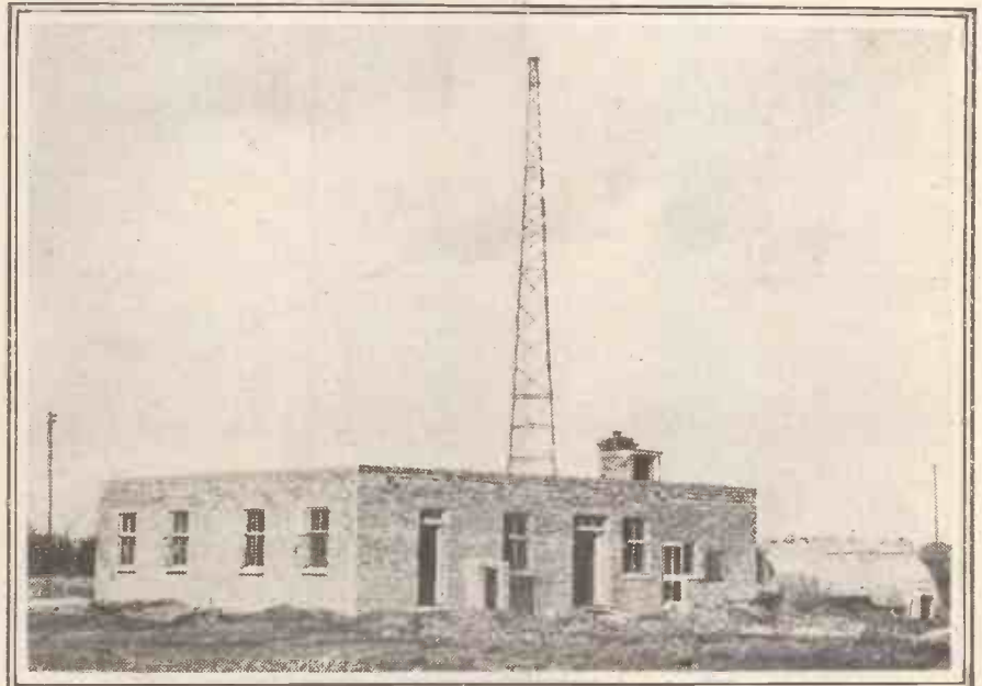
The Air Ministry's new wireless station at Mitcham, Surrey, which, as this photograph shows, is now nearing completion.
